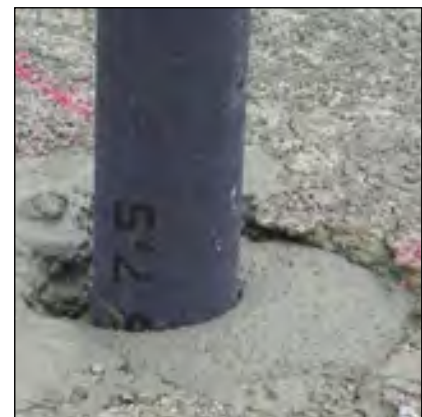
Visible return of sanded grout (118/7.5 pile)
